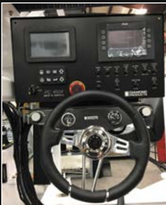
Centrally-located control station
